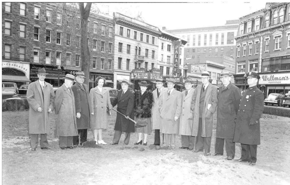
Advocate—Seat Construction of the Stamford Service Roll started this morning with Department of Service workmen, under the supervision of Councilman Ralph Rich, member of the Service Roll Committee, making the required excavation. A concrete foundation will be constructed. The work of preparing the slats which will bear the names of Stamford men and women in service is also being pushed as is the millwork for the monument at Stamford Trade School under the direction of Frank Laney. The committee on names, Col. James Wild, Kingsley Gillespie and Samuel Morrell, is seeking the names of all Stamford people in service at any time during the current conflict. Present in Central Park yesterday as ground was broken for the Service Roll were: Left to right—Dr. Charles E. Frange, Deputy Commissioner of Finance Frank C. Langley, Commissioner of Finance Frank T. Slavin, Mrs. Bindley Gillespie, Mayor Charles E. Moore, shown wielding the spade; Mrs. David Waterbury, sr., Corporation Counsel Charles N. Wexler, Kingsley Gillespie, City Engineer Leon C. Tuttle, Lieut. Col. James H. Wild and Patrolman Asa W. Scanlon, veteran of the World War I.
